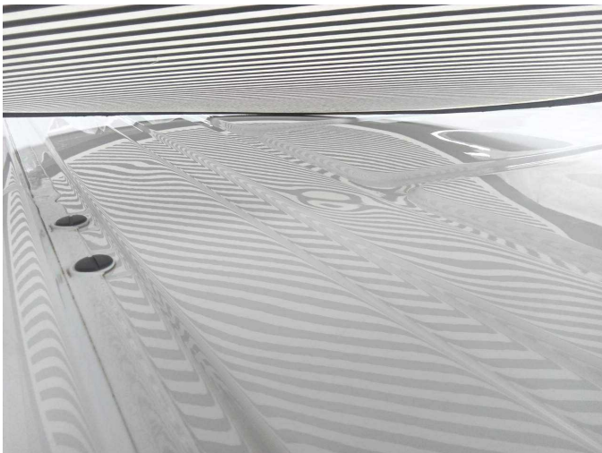
Damage 2: Roof: Roof (Grosse dellen gedrückt) - Deformed - Smooth repair work
