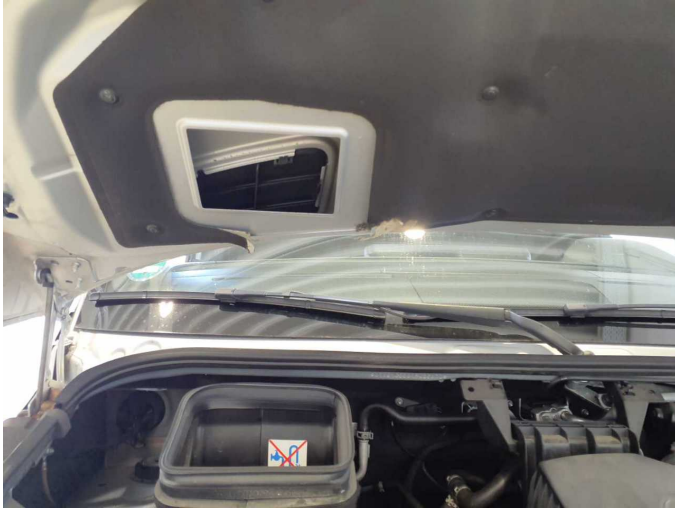
Damage 1: Bonnet: Insulation lining - Damaged - Replace
