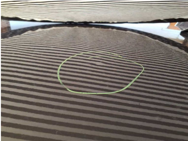
Damage #2: Roof: Roof - dent(s) - Smooth repair work
