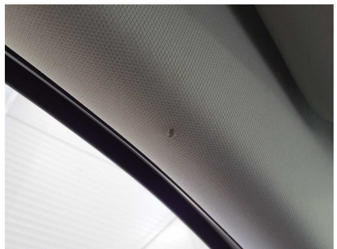
Damage 3: Trim / covers: Roof lining - Holes - Smart repair
