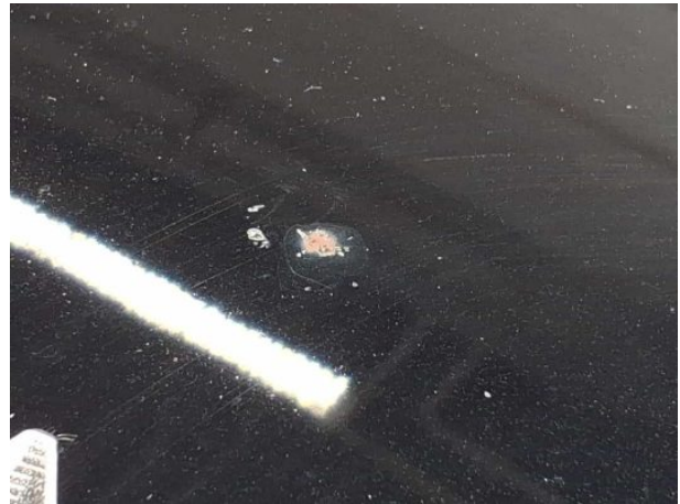
Damage #13: Roof: Roof - Corrosion - Repair and paint
