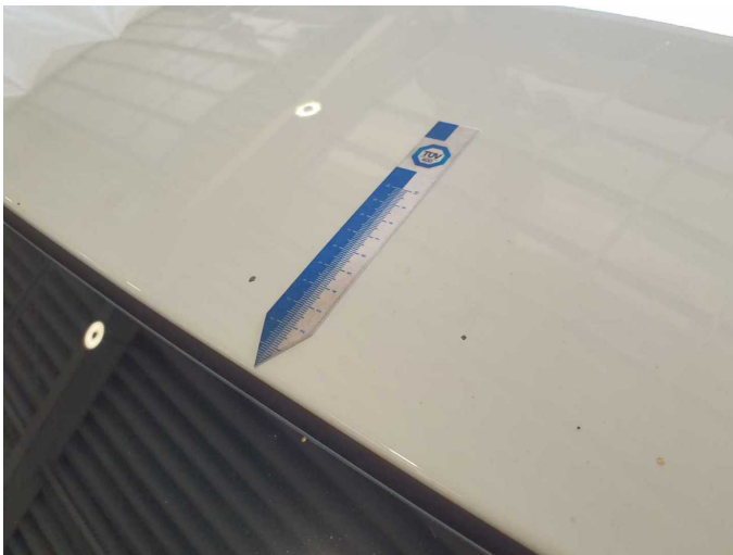
Damage 6: Roof: Roof (Wellig) - Paint defect - Repair and paint
