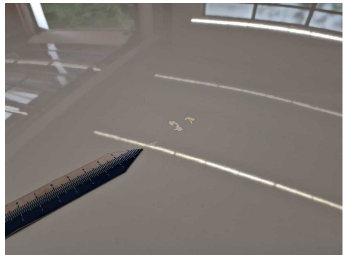
Damage 2: Roof: Roof - Soiled - Conditioning
