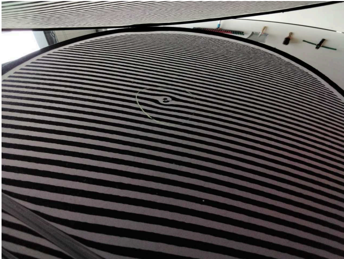
Damage 10: Roof: Roof - dent(s) - Smooth repair work
