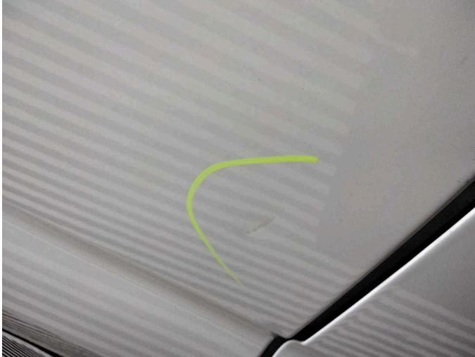
Damage 2: Sliding door, right: Sliding door - Dent / paintcoat damage - Repair and paint
