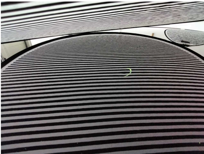
Damage 7: Roof: Roof - dent(s) - Smooth repair work
