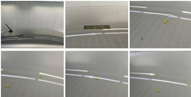
Roof, Hail damage, Paintless dent repair (hail)
