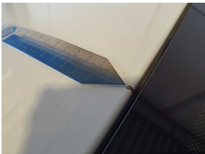
Damage 3: Roof: Roof (Dachkante) - Corrosion - Paint
