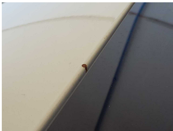
Damage 3: Roof: Roof (Dachkante) - Corrosion - Paint
