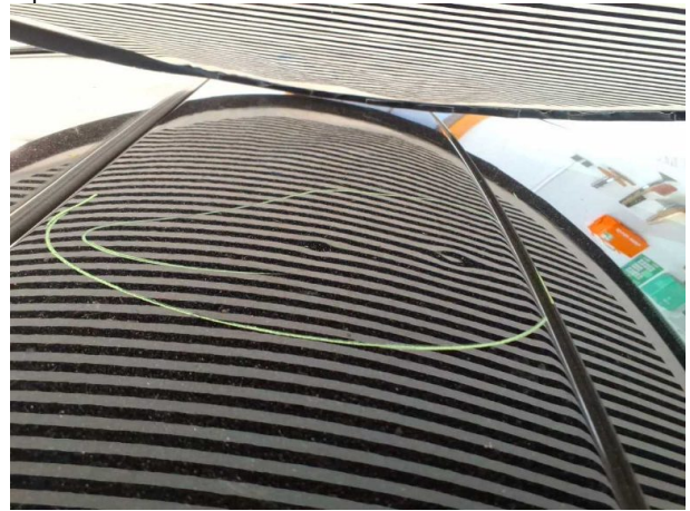
Damage #11: Roof: Roof - dent(s) - Smooth repair work
