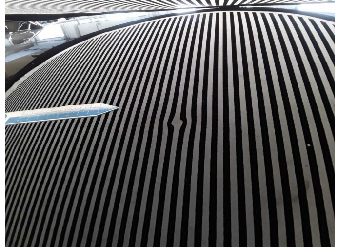
Damage 2: Roof: Roof - dent(s) - Smooth repair work
