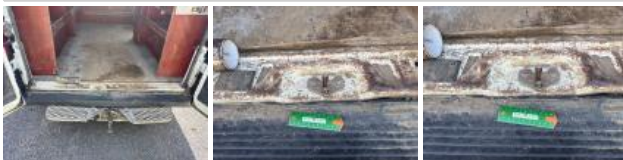
Jack, Missing, Repair/replace (lump sum)
