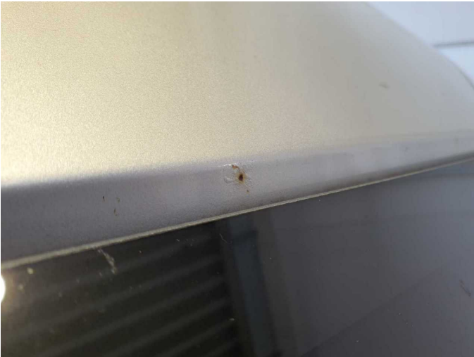
Damage 10: Roof: Roof (vorne) - Corrosion - Loss in value
