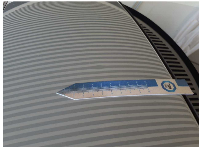
Damage 2: Roof: Roof - dent(s) - Smooth repair work
