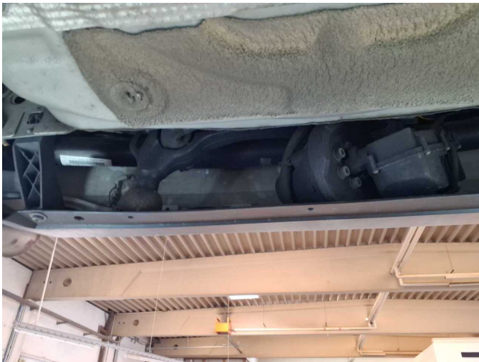
Damage 2: Rear bumper: Spoiler (Loch für anhängerkuppl. fehlt) - does not comply with manufacturer's specifications - Replace
