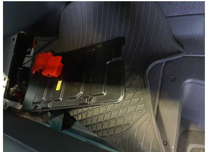
Damage 2: Electrical system: Battery (Tiefenentladen) - Functional / admissibility - Perform diagnosis
