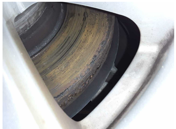
Damage 8: Braking system: Brake discs and brake pads - front (Verschlissen und) - Corrosion - Replace
