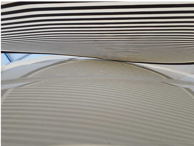
Damage 3: Roof: Roof - dent(s) - Smooth repair work
