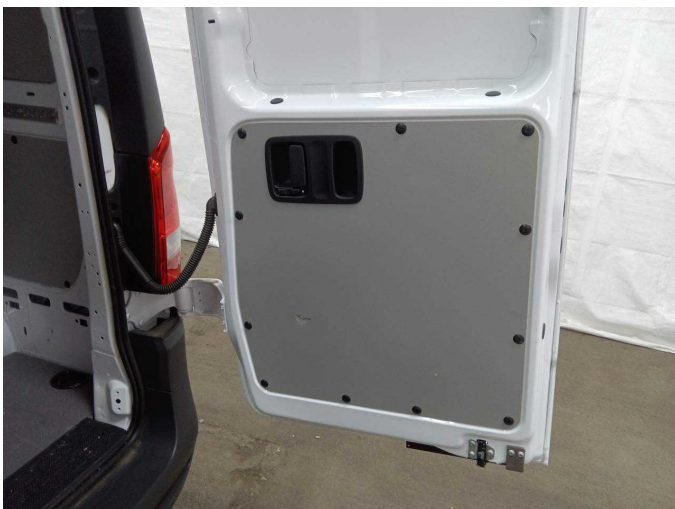
Damage 3: Trim / covers: Boot lid - interior trim - Holes - Replace
