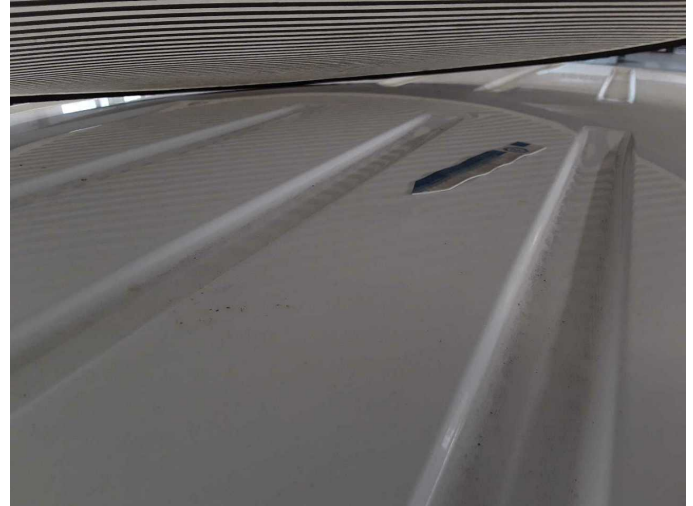
Damage 7: Roof: Roof - Deformed - Repair and paint
