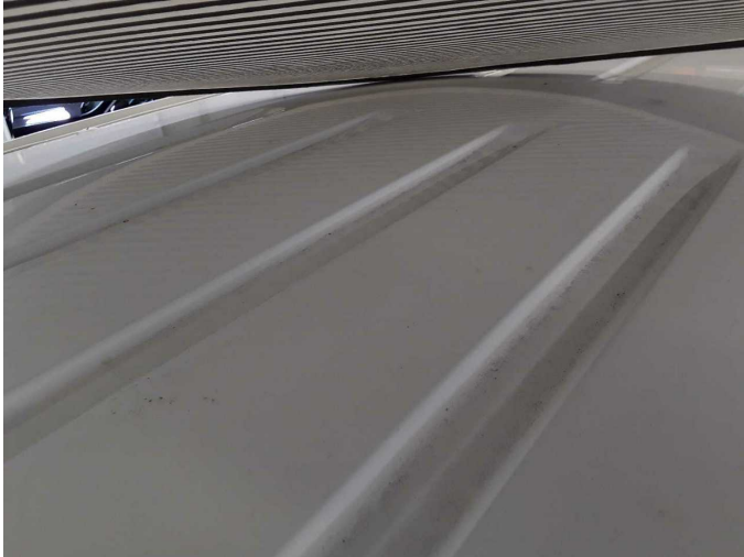
Damage 7: Roof: Roof - Deformed - Repair and paint
