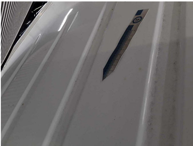
Damage 7: Roof: Roof - Deformed - Repair and paint
