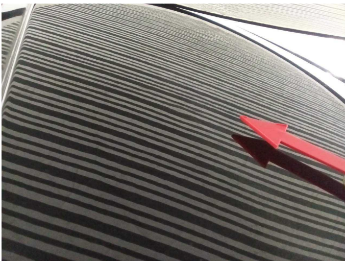
Damage 3: Roof: Roof - dent(s) - Smooth repair work
