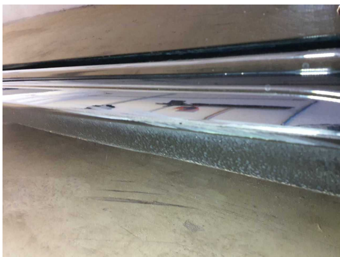
Damage 7: Sill - left side: Trim - Scratch(es) - Replace
