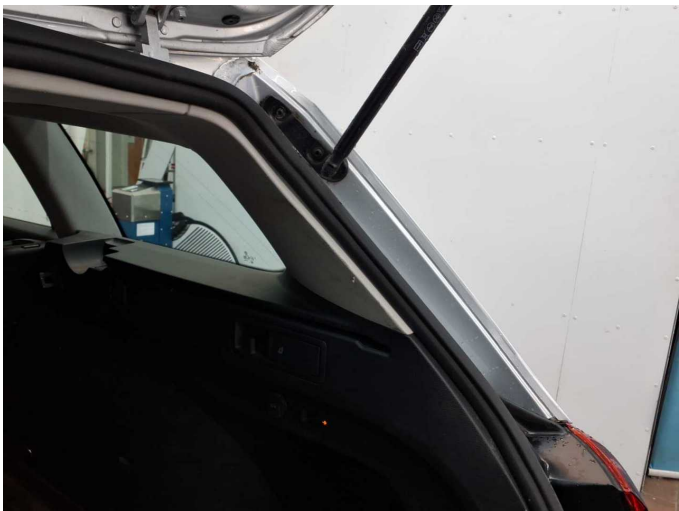
Damage 1: Interior: Interior - Scratch(es) - Loss in value
