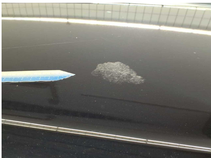
Damage 2: Roof: Roof - Soiled - Conditioning
