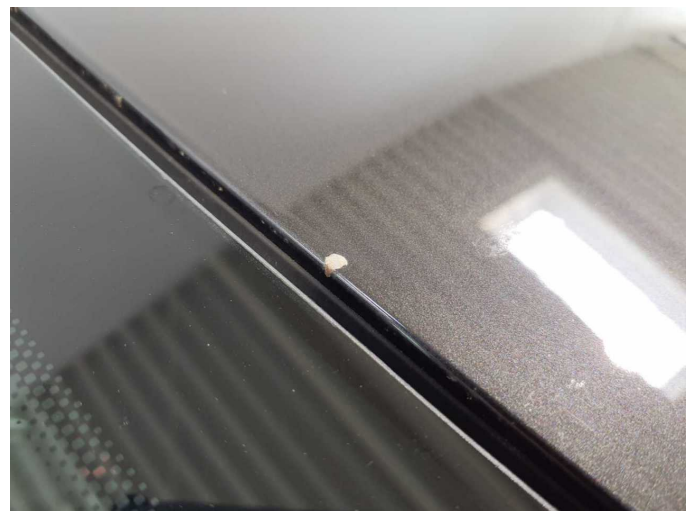
Damage 15: Roof: Roof - Corrosion - Repair and paint
