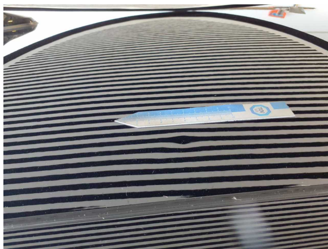
Damage 1: Roof: Roof - dent(s) - Smooth repair work
