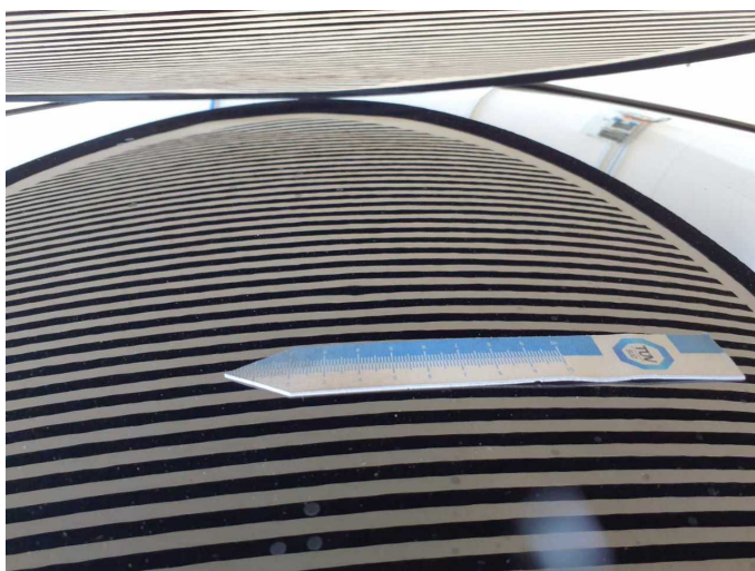
Damage 1: Roof: Roof - dent(s) - Smooth repair work
