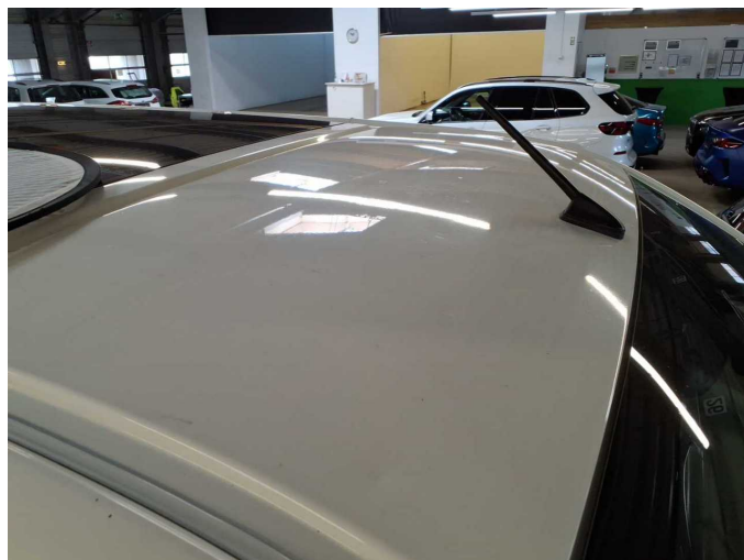
Damage 19: Roof: Roof - Dent / paintcoat damage - Paint
