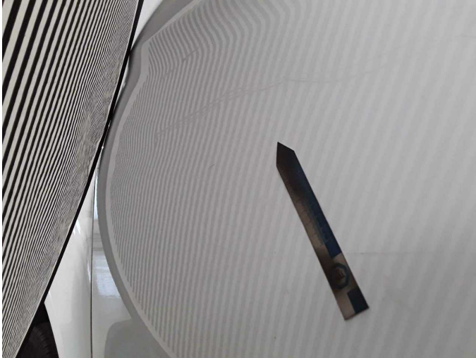
Damage 9: Sliding door, right: Sliding door with glass panel - Dent / paintcoat damage - Repair and paint
