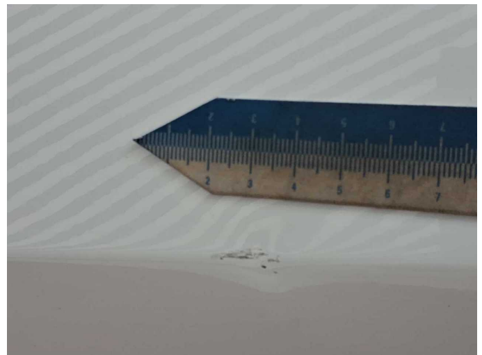
Damage 6: Sliding door - left side: Sliding door with glass panel - Dent / paintcoat damage - Smart repair
