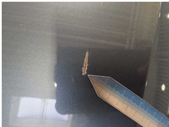
Damage 13: Bonnet: Bonnet - Corrosion - Repair and paint
