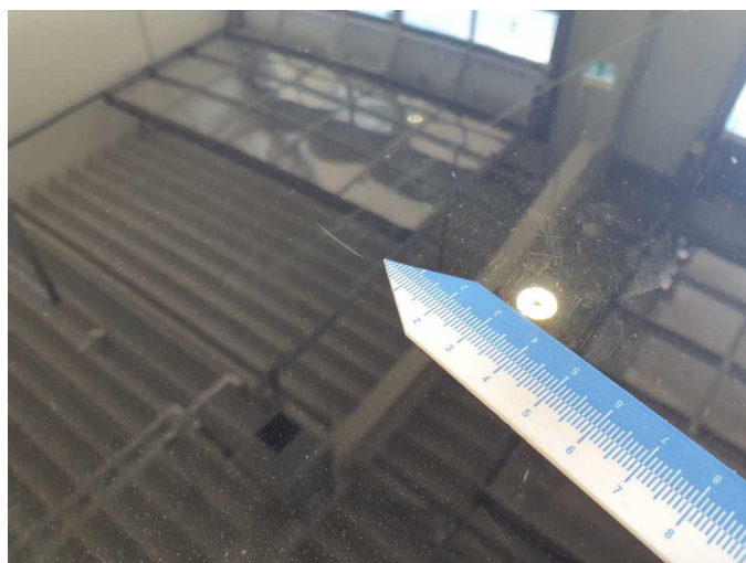
Wear and tear 3: Roof: Roof (polierbar) - Scratch(es) - No deduction
