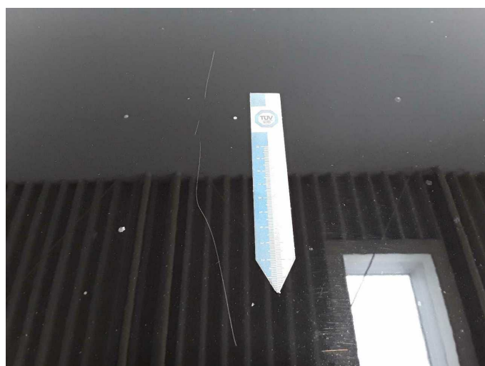
Damage 7: Roof: Roof - Scratch(es) - Paint
