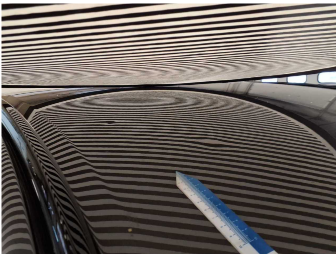
Damage 4: Roof: Roof - dent(s) - Smooth repair work
