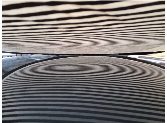
Damage 13: Roof: Roof - Damage by hail - Smooth repair work
