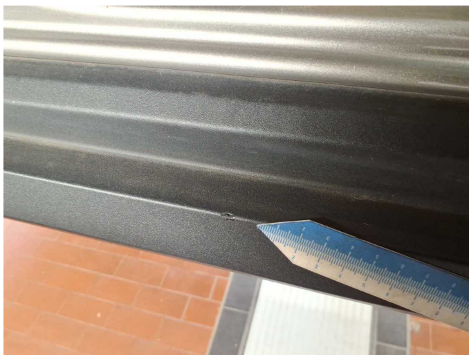
Wear and tear 2: Sill - right side: Trim - Scratched - No deduction
