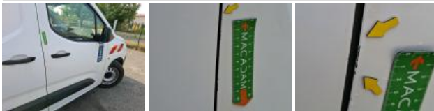
Roof, Rust, Paint
