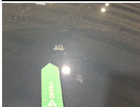
Roof / - / Paint etching
