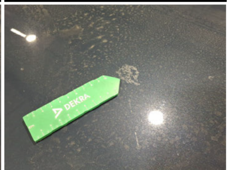
Roof / - / Paint etching
