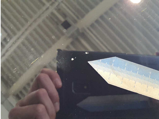
Damage 5: Roof: Roof - Stone chips - Paint
