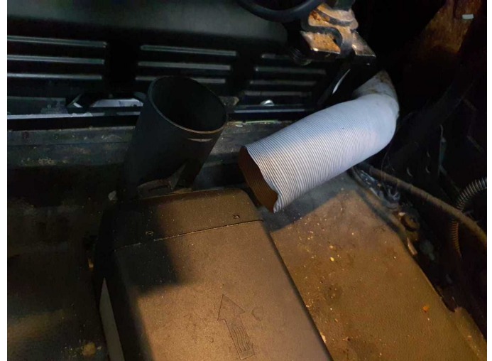
Damage 4: Heating system: Auxiliary heating (Schlauch abgezogen) - Functional / admissibility - Perform diagnosis
