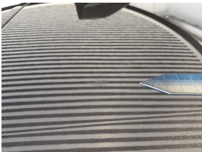
Damage 14: Roof: Roof - Paint defect - Repair and paint
