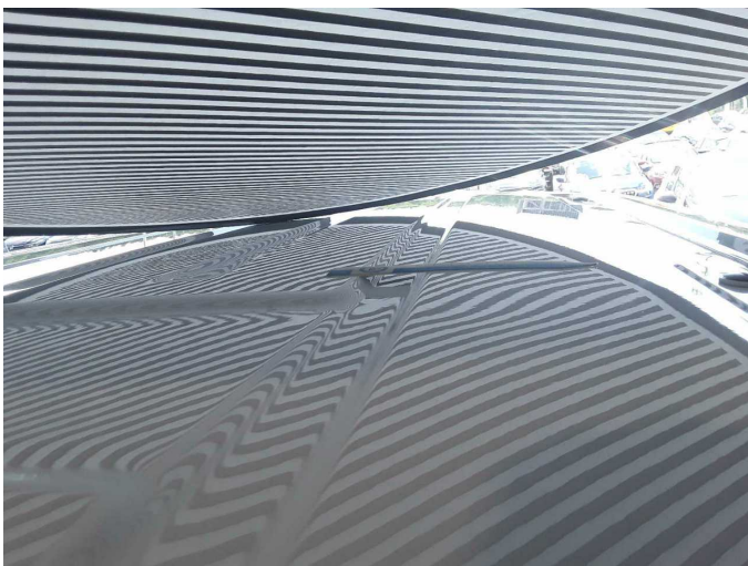
Damage 3: Roof: Roof - dent(s) - Smart repair
