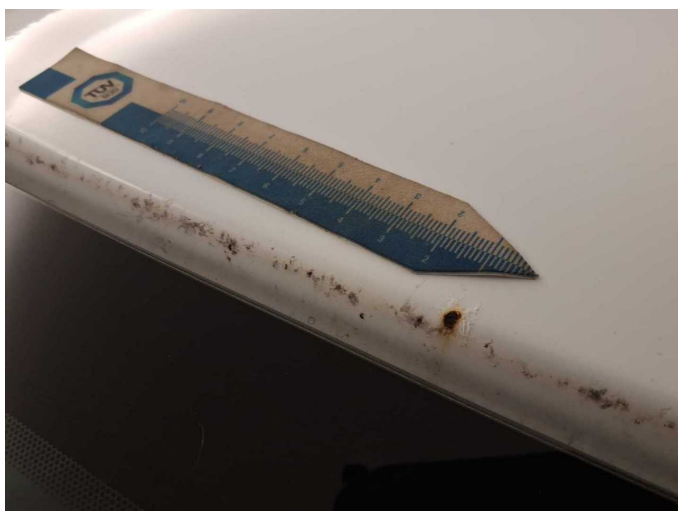
Damage 7: Roof: Roof - Corrosion - Paint
