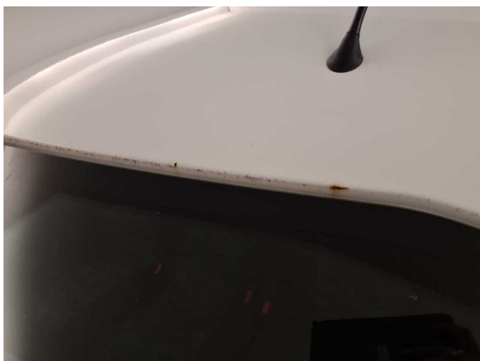
Damage 7: Roof: Roof - Corrosion - Paint
