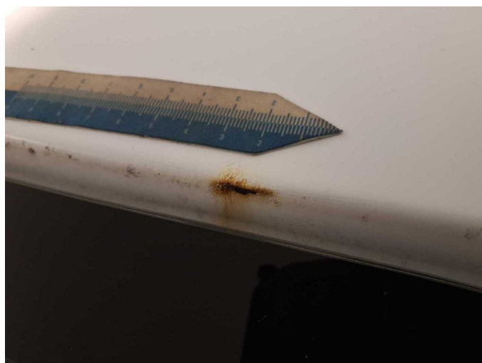
Damage 7: Roof: Roof - Corrosion - Paint
