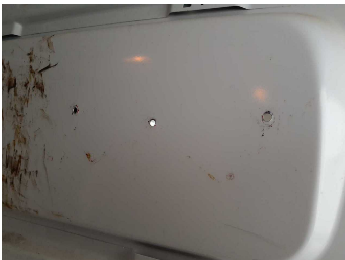
Damage 13: Body: Partition wall - Holes - Replace
