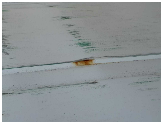
Damage 8: Roof: Roof (beschädigt) - Corrosion - repair according to calculation
