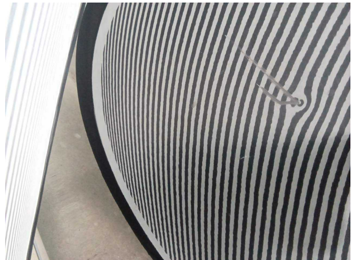
Damage 5: Sliding door - left side: Sliding door - Dent / paintcoat damage - Repair and paint
