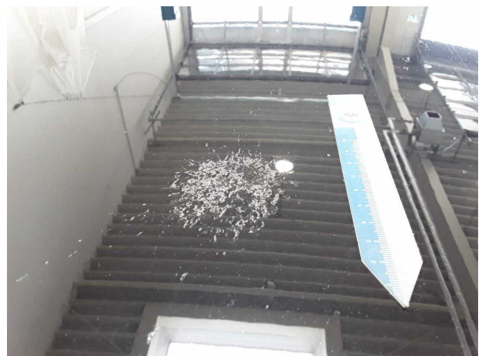
Damage 2: Roof: Roof (Anätzung) - Paint defect - Repair and paint
