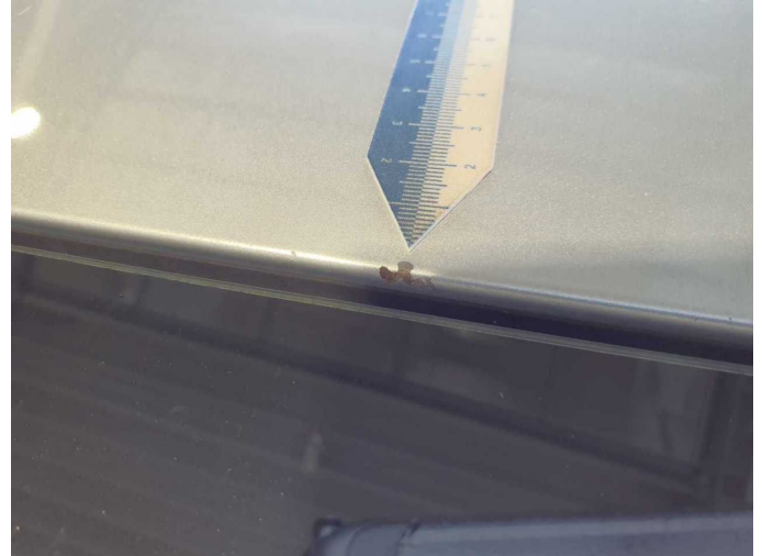
Damage 12: Roof: Roof (+ Kratzer) - Corrosion - Paint
